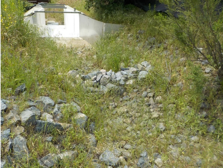
Figure 7. Erosion control at OF008 (Armoring)
