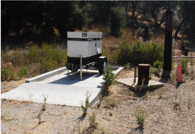
Figure 9. New ELV Generator
