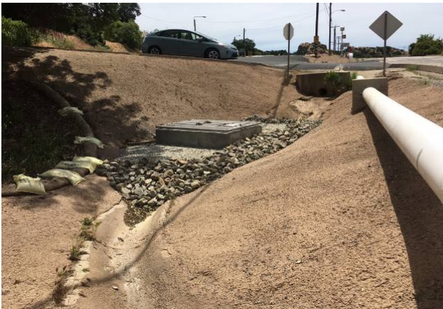
2017: Upper Parking Lot Media Filter
