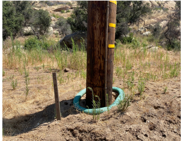
2020: Southern Buffer Zone Utility Pole BMPs
