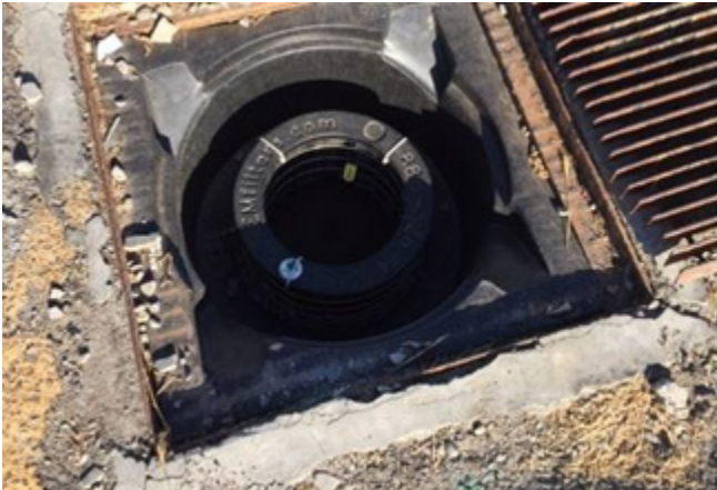
2017: Administration Area Inlet Filters (Filter Basket)
