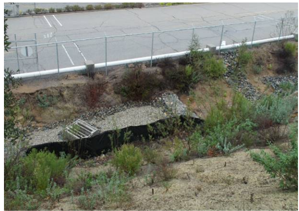
2012: B-1 Sedimentation Basin and Media Filter
