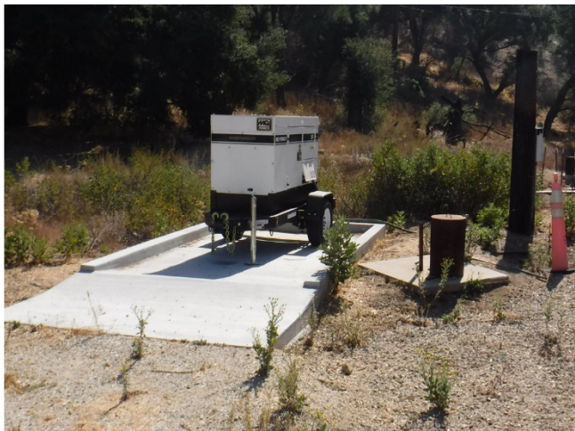
2020: Outfall 009 ELV and Biofilter Cistern Generators Added
