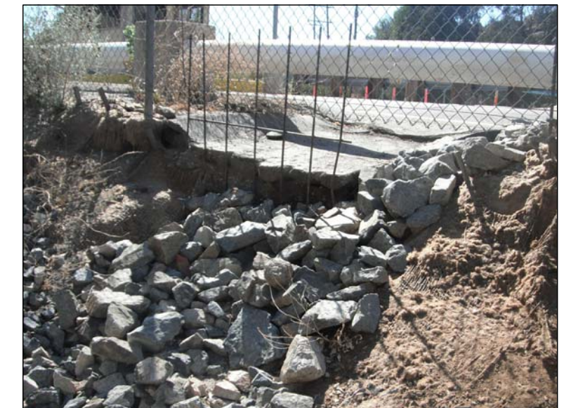
PHOTO #2: LOOKING NORTHWEST AT RIPRAP INSTALLED AFTER EXISTING CURB CUT. THIS DESIGN IS RECOMMENDED FOR THE (3) 36" PROPOSED CURB CUTS.
