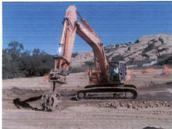
Compacting soil in berm of the temporary sediment control BMP in the B1-2 ISRA area.
