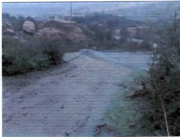
Water bar on access road to CTLI-1 ISRA areas.
