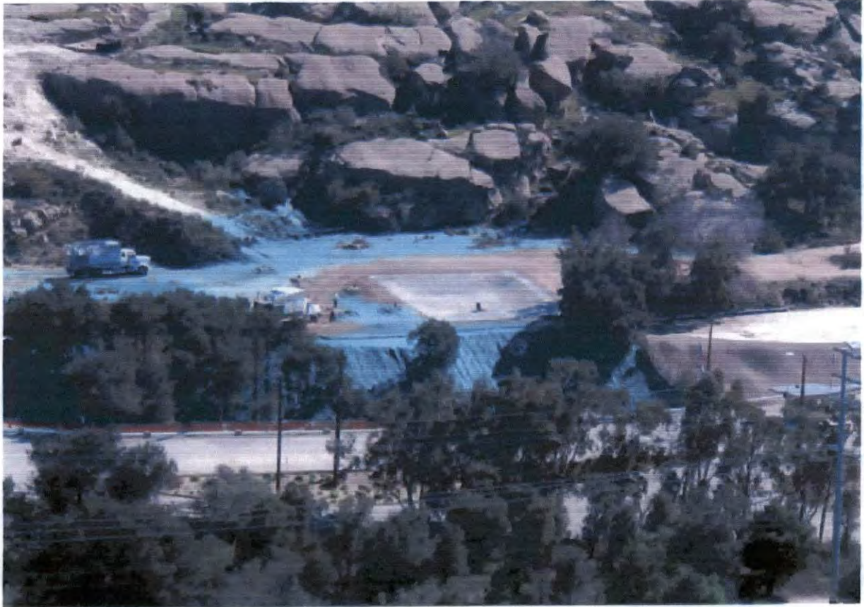
Restoration of B1-2 ISRA area near completion, including installation of temporary sediment control BMP and application of hydroseed mulch.
