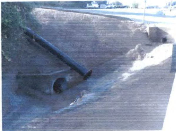
Piped discharge from B1-2 retention pond into culvert leading to Northern Drainage (2/26/11).
