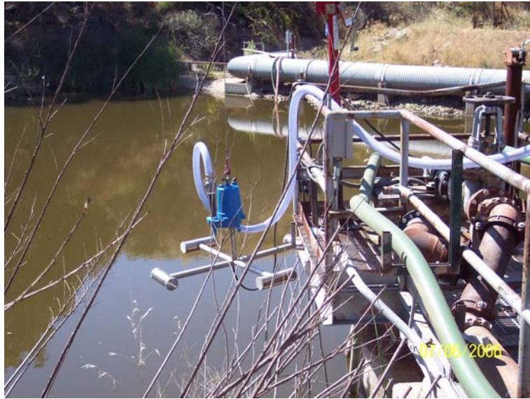
Figure 4 Pump and Manifold
