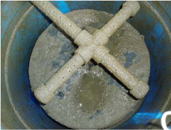
Clogged Peat Moss (7/28/06)
