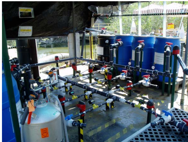
R2-A Pond Filtration Pilot Test: Looking South
