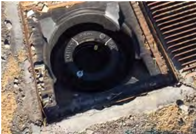
2017: Administration Area Inlet Filters (Filter Basket)
