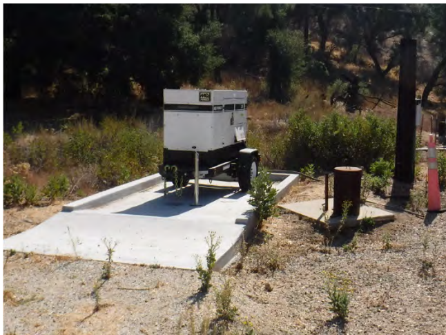
2020: Outfall 009 ELV and Biofilter Cistern Generators Added
