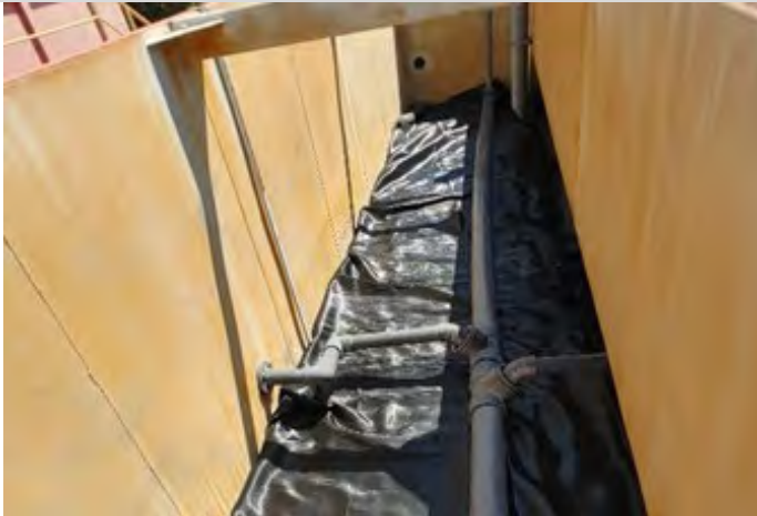
Figure 6. Reconstructed ELV Media Bed Showing Flow Distributing Geotextile on Top of Media
