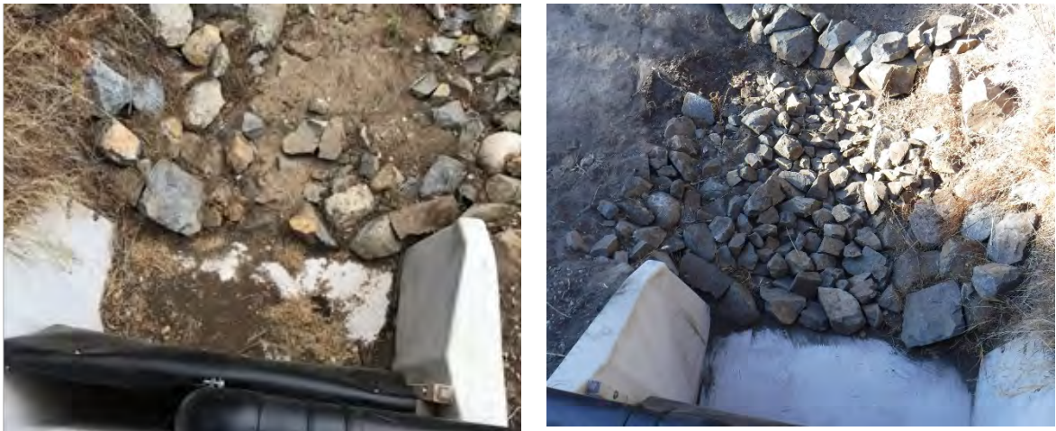
Figure 7. Check dam and ponding area upstream of CM-4 before (left) and after (right) reconstruction
