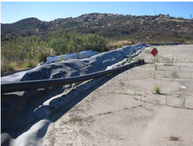
2011: Helipad Berms and Pumps
