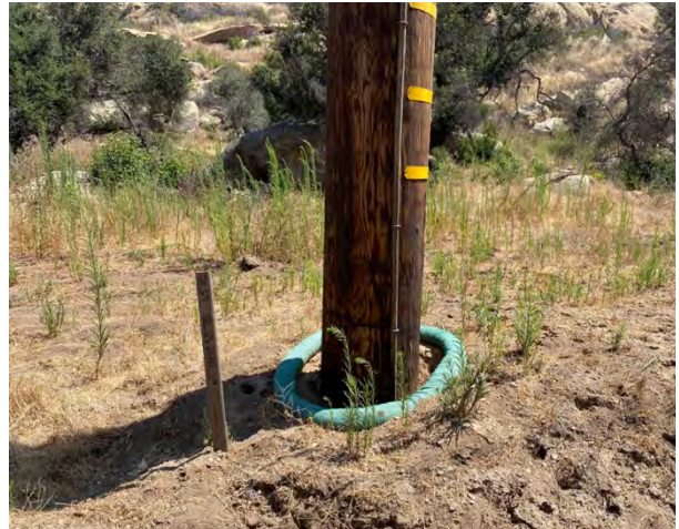
2020: Southern Buffer Zone Utility Pole BMPs
